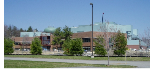
"Green Construction" - A view of BMS's lab/office building & manufacturing blg. under construction at the site.
